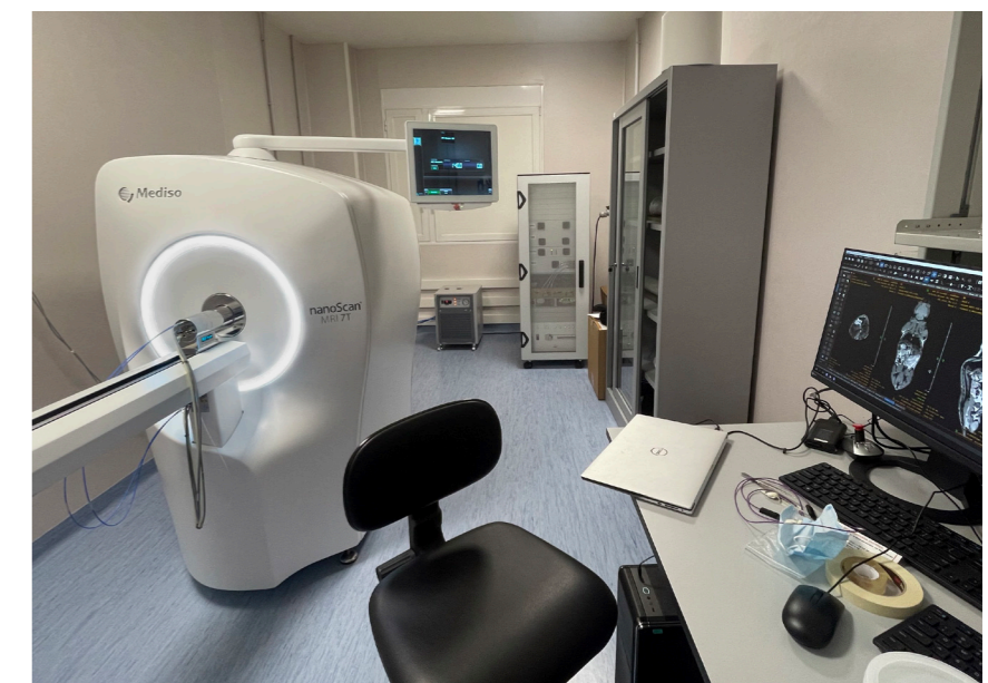
nanoScan® MRI 7T reference installation with every system component (magnet, workstation, electronic cabinet, He-compressor, chiller) located in the same imaging room.
